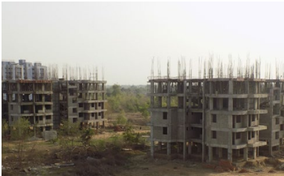
C type Quarters (Capacity: 56 units) 40% complete(RCC of 5 th floor is in progress)
